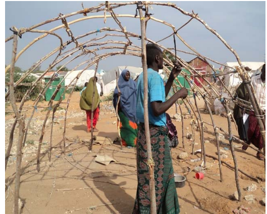
IDPs constructing new shelters in Mogadishu. Credit: Save Somali Women, Children (SSWC)
